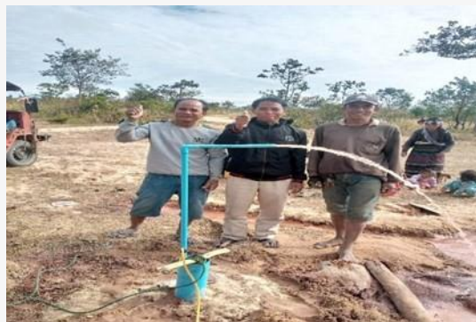
Water coming out from the installed pipes. Praise God! Photo taken by Daniel Yang)
