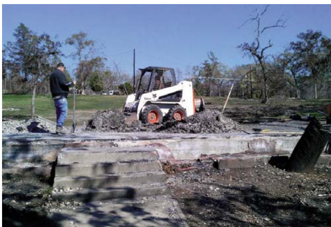
Glen Grant and local volunteer Carol Nokota, operating the skidsteer at a residence demolished by the fire.
