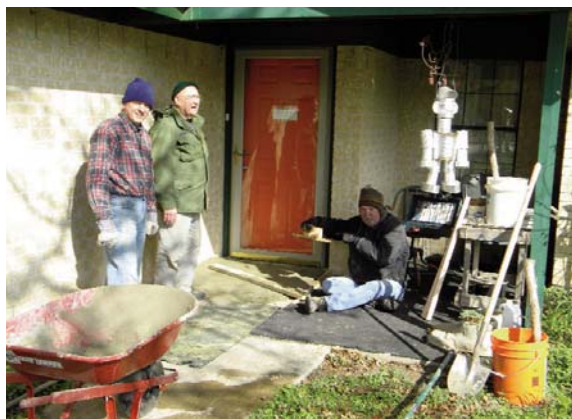
Left to right: David Gingles, Glenn Dutton, and Team Leader Glen Grant using a homemade trowel to finish work on a wheelchair ramp.
