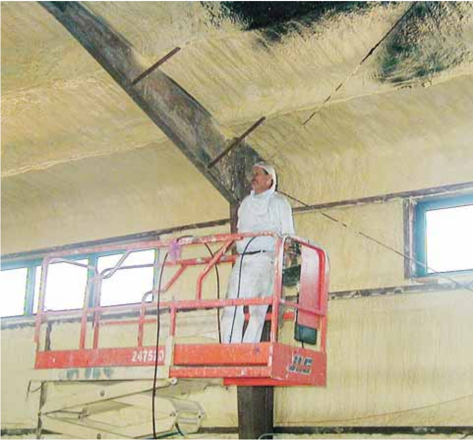
Using a mechanical lift, a volunteer surveys the work yet to be done on the suspended ceiling in Youth for Christ Center.
