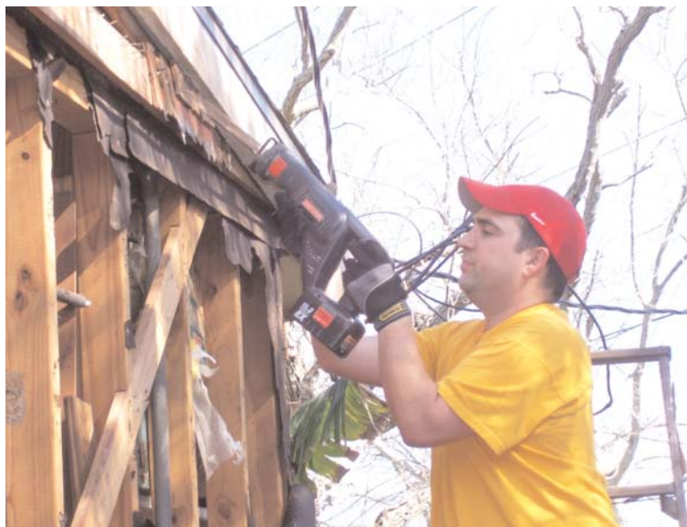
Jim Schwartz works on the exterior frame of a home in the Galveston area.
