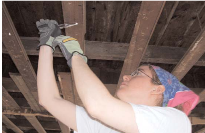
Jennifer Schwartz repairs beams in the ceiling of a house damaged by Hurricane Ike.
