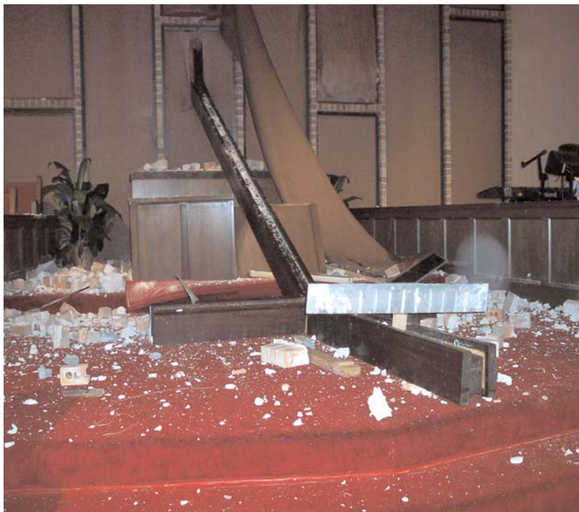
The United Methodist Temple memorial cross and back wall of the sanctuary was destroyed by Hurricane Rita in 2005.
