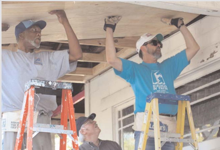
Homeowner, Gary Thompson and East District Superintendent, Rev. Keith Whitaker place new plywood on the ceiling.
