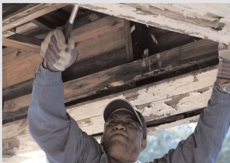
Rev. Earl Bledsoe, West District Superintendent removes rotted wood from the ceiling in the home of Debra and Gary Thompson.
