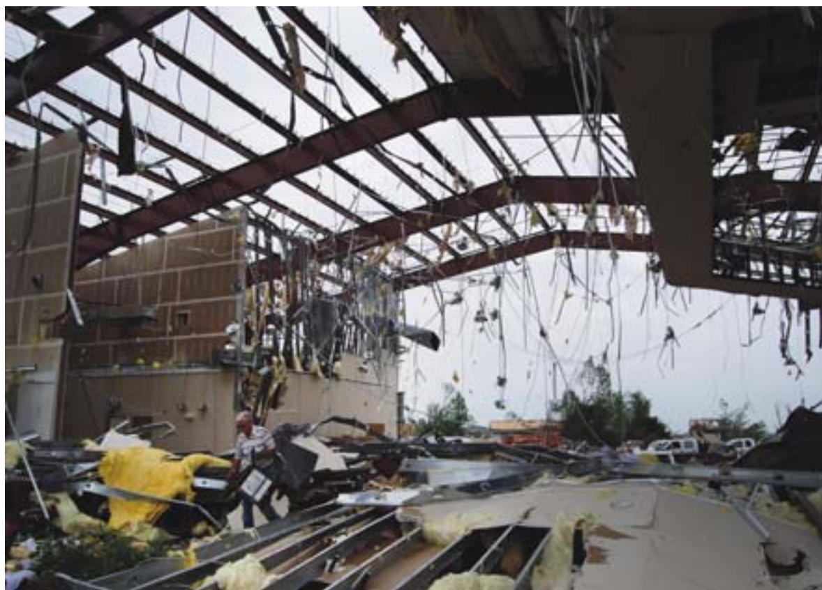
An interior view of St. Paul’s UMC shows the bare support beams, which are still standing following the tornado in Joplin, Missouri. Early Responders train for such a time as this.
