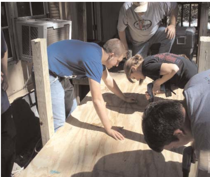
One ramp on its way. Youth began work on a wheel chair ramp for a Linden resident.
