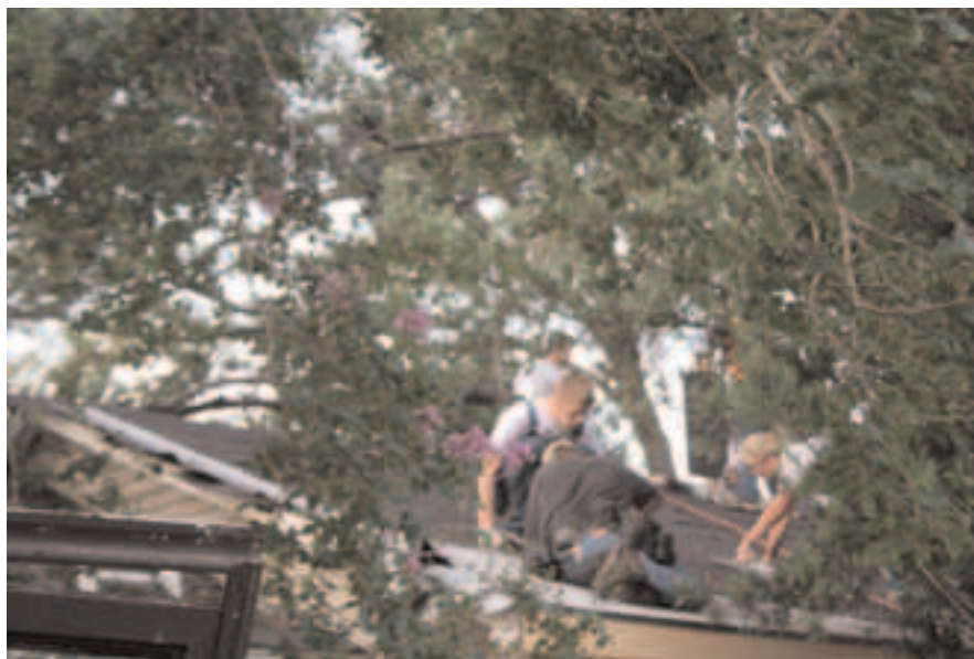
Volunteer workers in the Beaumont area began repairs on the roof of a house damaged by Hurricane Rita.
