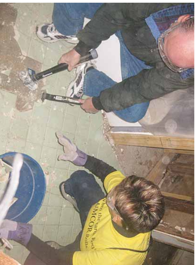
Top Left Photo: Verronda Flanagan takes a break from registering Ike volunteers to knock out drywall.
