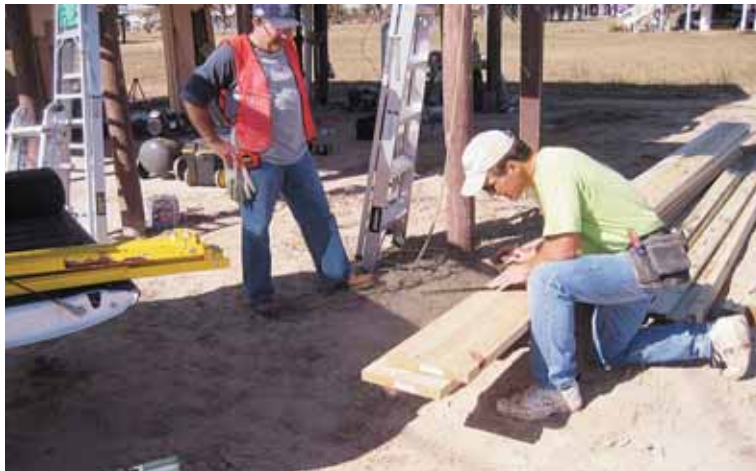
Ralph Hendricks and Tim McGuire from Lake Jackson, renovated the damaged steps at the nearby house in Corpus Christi, Texas.
